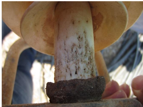
Fig. 4. Pinholes due to corona discharges on a PTFE composite insulator
